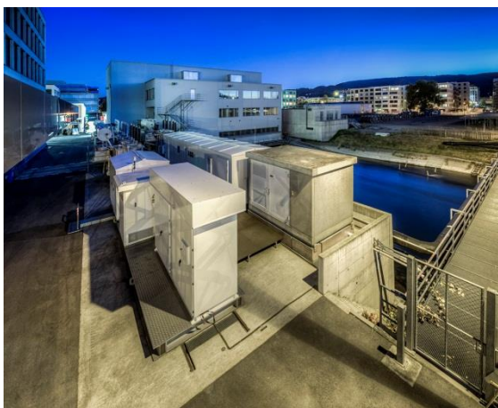
Figure 6 The Zurich BESS
