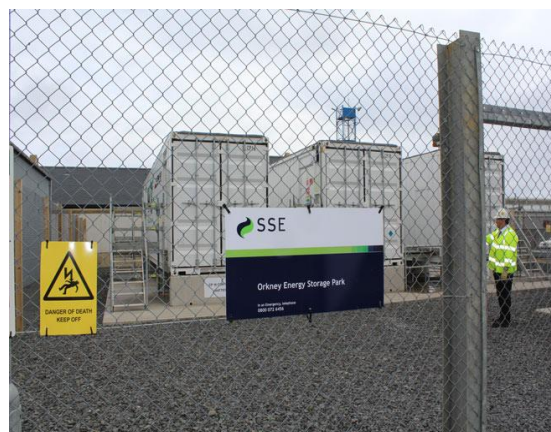
Figure 8 The Orkney Storage Park project
