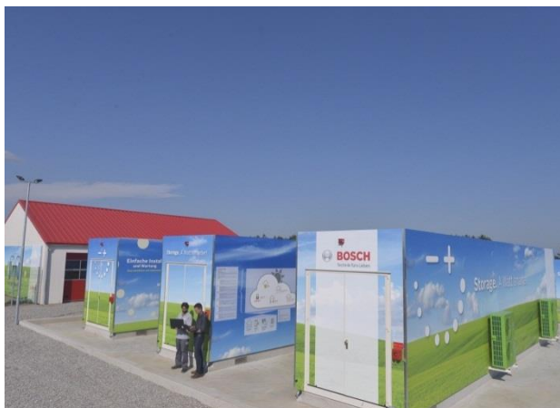
Figure 7 Bosch Braderup ES Facility
